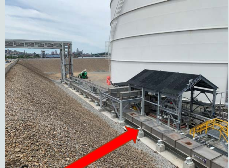
Shrouding at LNG process area next to LNG storage tank
